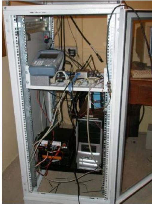
FIGURE 3.14: The cabinet where the receiver placed.
