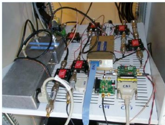
FIGURE 3.16: The filtering and amplification unit at the closet of the receiver.
