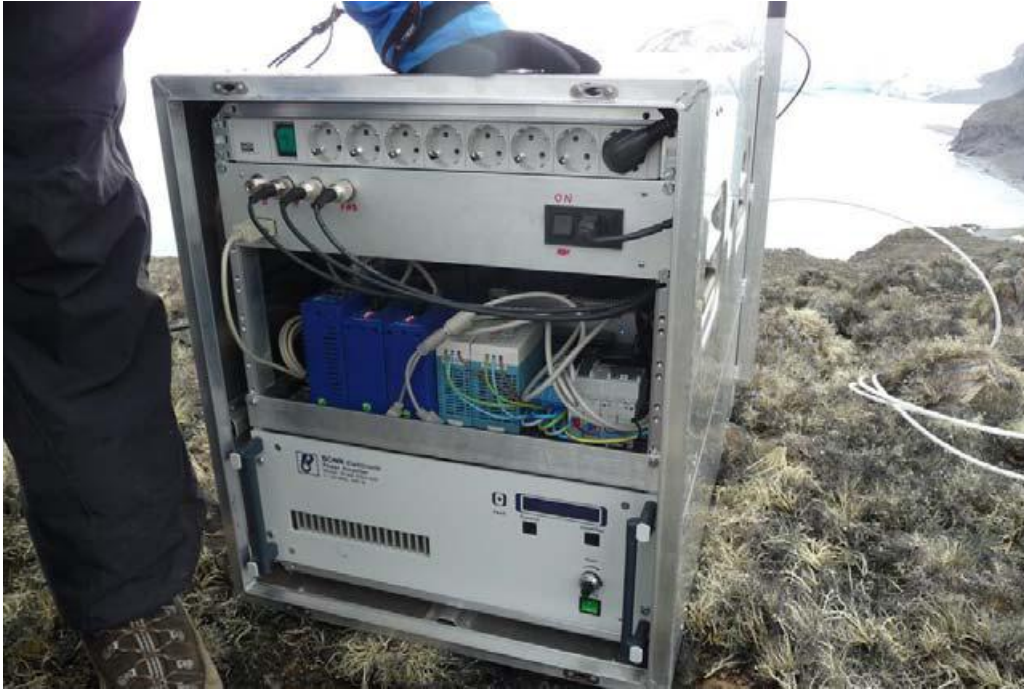
FIGURE 3.9: Front view of the waterproof sealed box.
