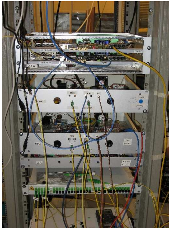
Fig. 4. 14 - SARDANA rack with two ONU prototypes: ONU layer 2 (above) and opto-electrical ONUs layer 1 (middle) subsystem
