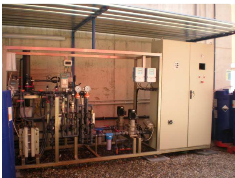
Figure 5.2. Picture of the ED pilot plant located at the El Prat Seawater Desalination Plant.
