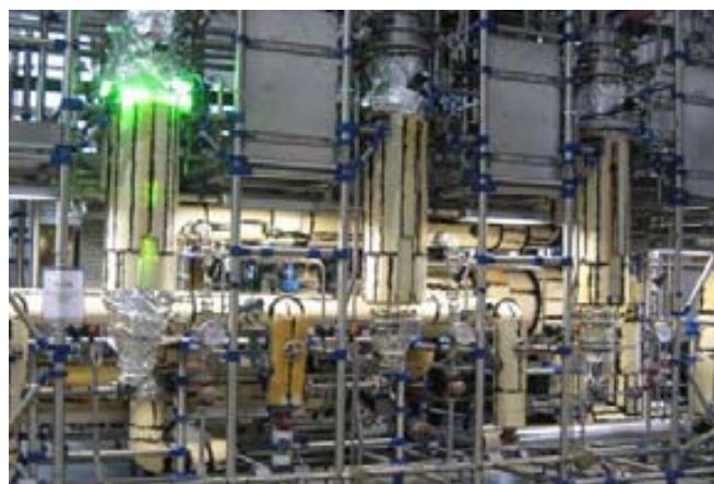
Figure 40. Sanofi photochemical facilities with three photochemical reactors.
