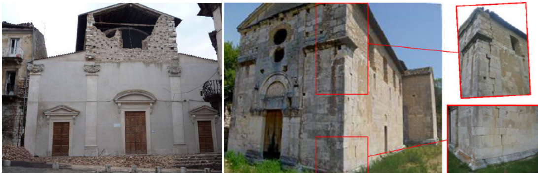
c) Collapse of the gable of San Biago church (Brandonisio et al., 2013) d) overturning of façade of San Paolo a Peltuinum church (Brandonisio et al., 2013)
