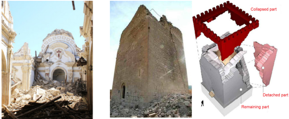
a) Collapse of the transept of Santiago church (Romao et al., 2013) b) Damage of Espolón tower (adapted from Feriche et al., 2012)
