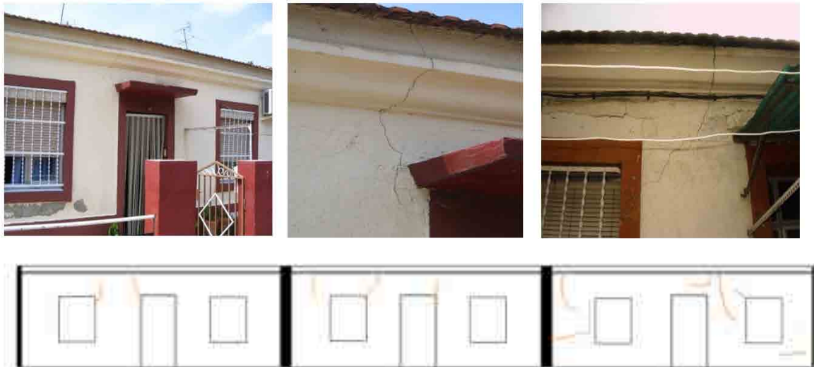
Figure 2.15. Photographs of damage occurred in buildings due to tunneling (three last dwellings).
