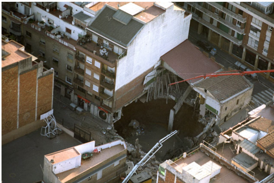
Figure 1.1. Ground collapse in the neighborhood of 'El Carmel' (Barcelona) Source: El Periódico de Catalunya.
