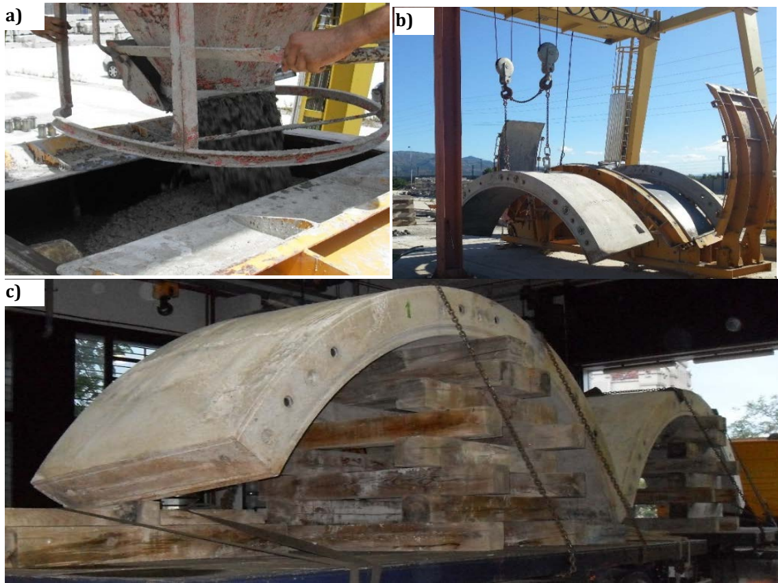
Figure 4.12 Concrete pouring a), unmoulding operation b), and transport c) of the segments
