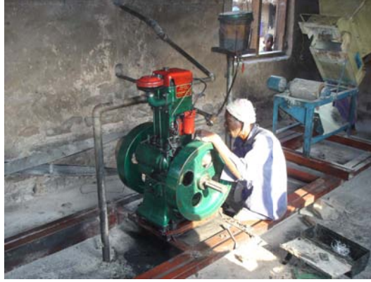
Figure 8.9: Worker in a MFP, in Seneso. In the picture, the diesel engine and the cassava grater. Source: Pol Arranz-Piera.
