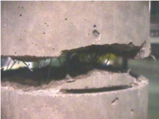
Figure 2.6. Failure outside the notch plane
