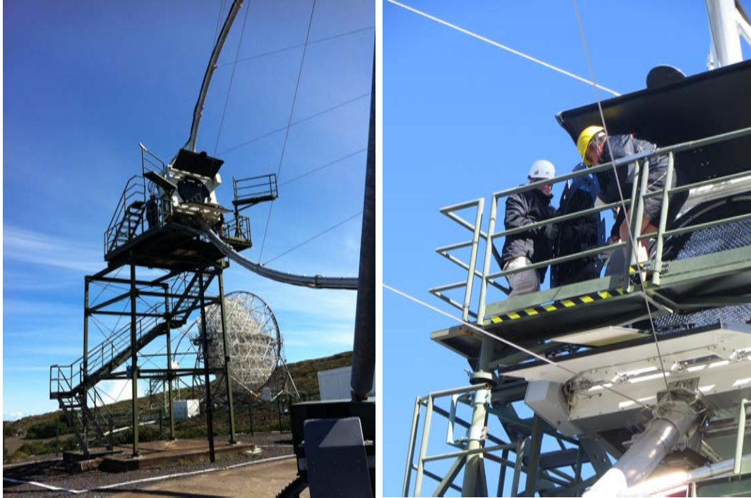
Figure 4.19: The filters are installed from the front of the camera, which can be accessed from a bridge that is part of the camera tower. The mounting is a task for two people, that carry the filters frame to the bridge and screw it to the camera.
