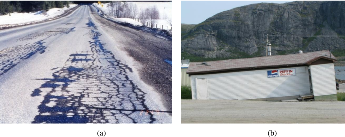
Figure 1.1 (a) Freeze-thaw damage on pavements ( http://www.pavementinteractive.org/frost-action/ ); (b) Thaw settlement of building at Nain, Labrador ( https://ipa.arcticportal.org/news/ )
