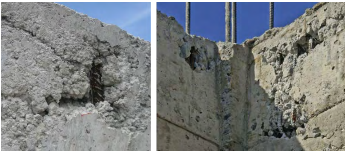
Figure 1.4. Exposed reinforcement caused by casting with concrete of inadequate slump
