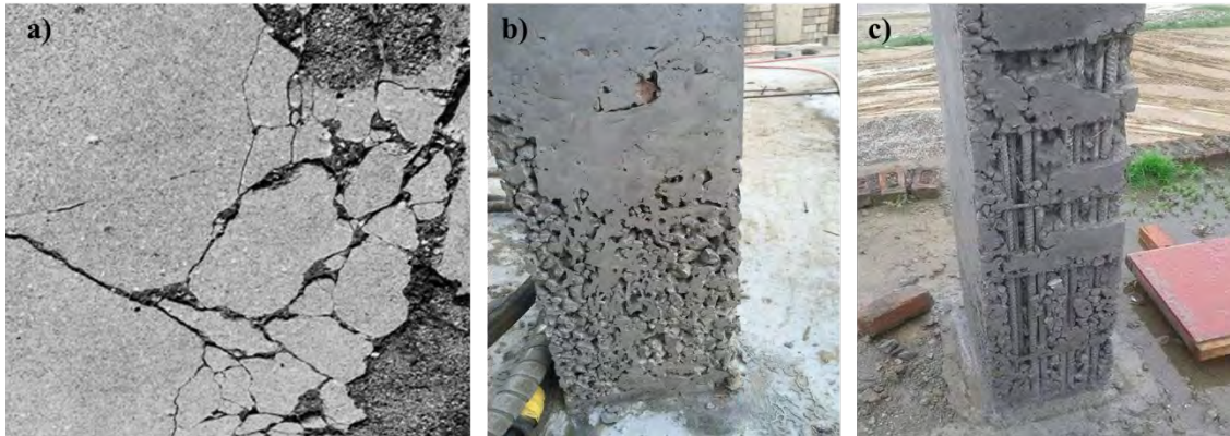
Figure 1.19. Typical damages generated by segregation of fresh concrete; a) delamination of concrete floors surface; b) aesthetics deficiencies in vertical applications; c) exposed reinforcement in pillars
