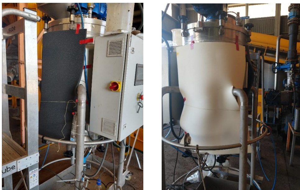
Figure 68: Reactor insulated with foam.
