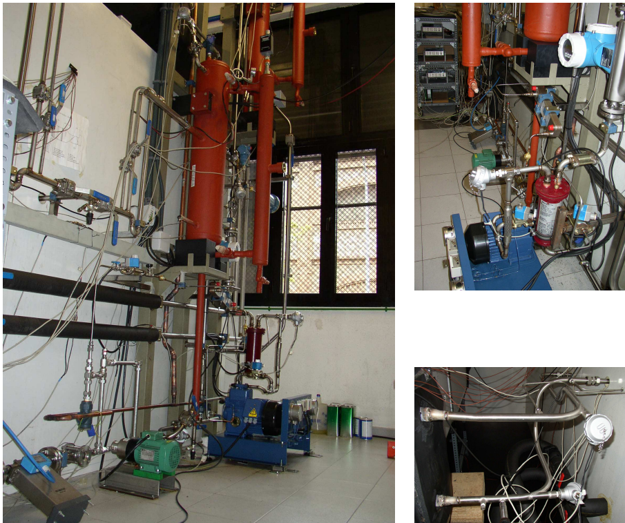
Figure 4.4: Liquid overfeed facility. Left: overfeed ref. circuit (LPR, comp, pump) Right: details of compressor and evaporator connection.[2]
