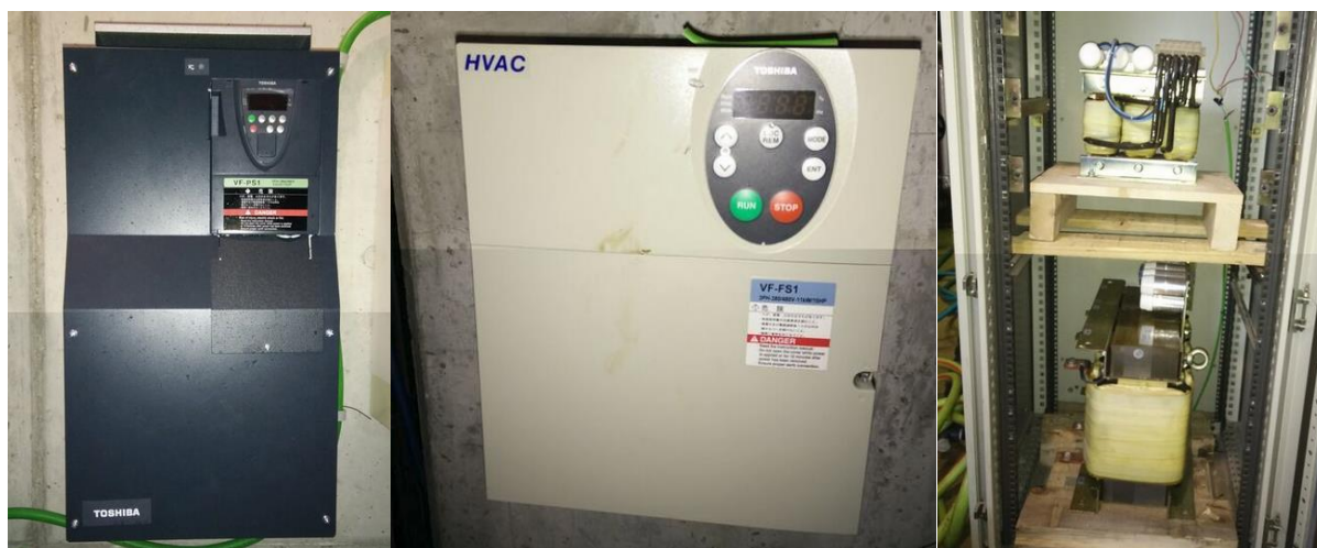
Figure 6.13. Frequency drivers (left and centre) and wave filters (right).
