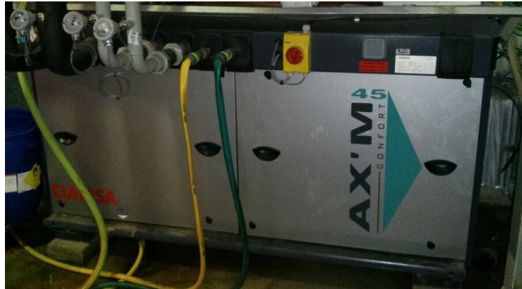
Figure 4.3. Air handling unit.
