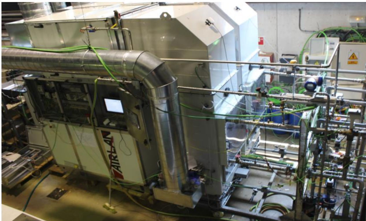
Figure 6.1. Picture of the hybrid liquid desiccant system during its set-up phase in Tarragona.
