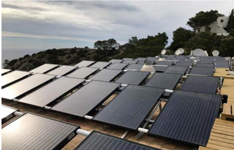
Figure 2-12. Covered PV/T collectors in Spain (EndeF Spanish manufacturer) [105].
