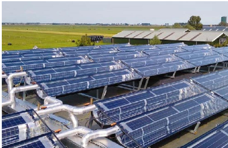
Figure 2-14. LCPV/T system in north Holland for food industry (Solarus) [107].
