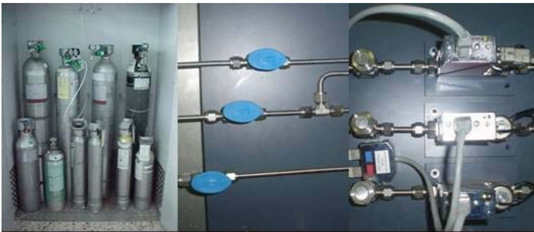
Figure 5.5: Gas flow system: Gases stored in bottles under high pressure (left); Gas transport system and manual valves (center); Mass-flow controllers (right).
