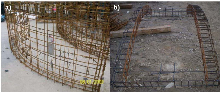
Fig. 8. Reinforcement cages for the precast segments: (a) PS-50 and (b) optimized RC-SFRC segment.
