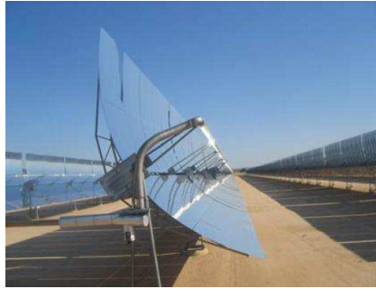
Figure 1.5: Structure and mirrors at a SEGS solar plant [12]
