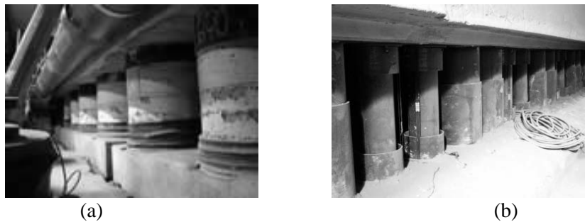
Figure 2.17. Example of modular yielding supports (slots and springs) installed in the interface vault-invert of tunnels excavated through swelling rocks: (a) highly deformable concrete springs (Solexperts HDC®) in Chienberg tunnel (Jura Mountains); (b) metallic springs in a circular test section of Lilla tunnel (Lower Ebro Basin) (after Berdugo, 2007)
