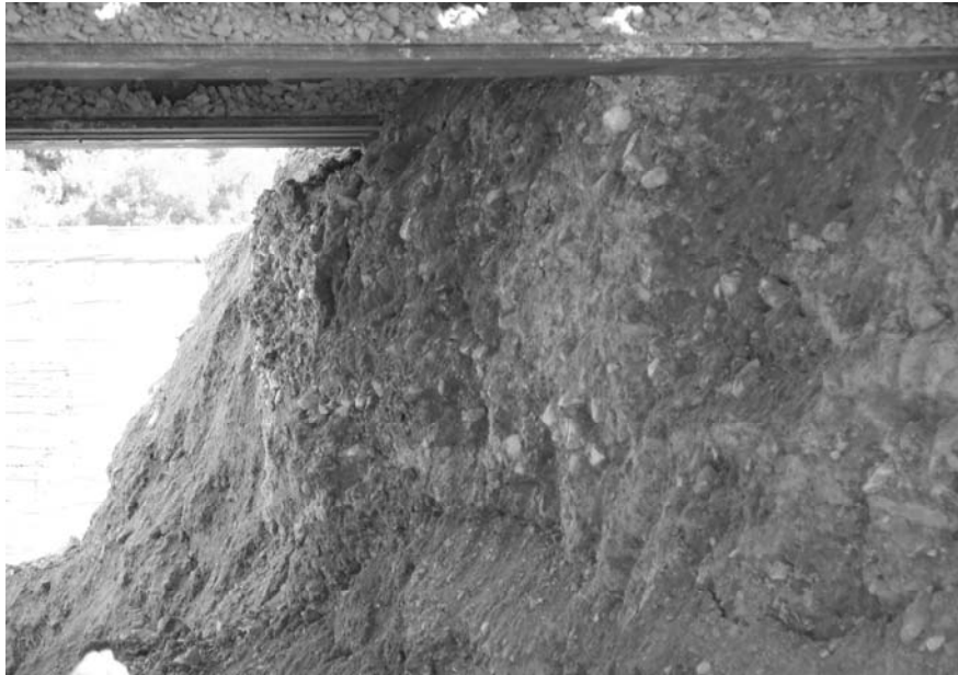
Figure 8.17. View of a cut across one of the embankments made during underpinning operations. Two jet-grouting columns as well as a level of cement treated material, in the lower part, are visible.
