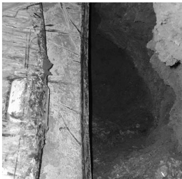
Figure 5.2. Caverns encountered during excavation with open shield through massive gypsum in Madrid.
