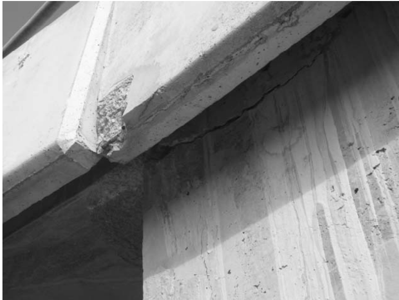
Figure 8.14. Damage observed near abutments
