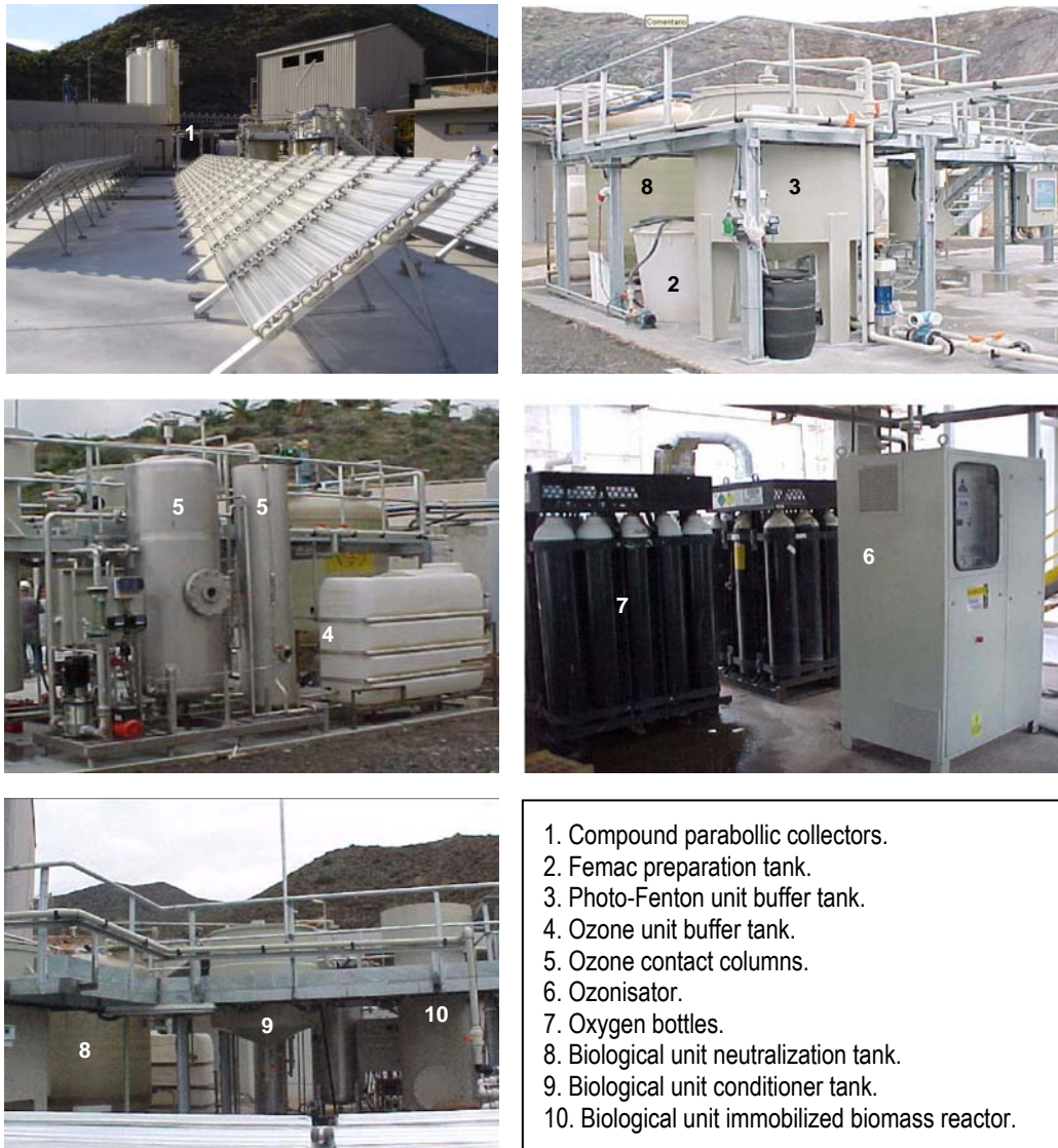
Figure 6.3. Images of the CADOX demonstration plant installed in DSM Deretil.
