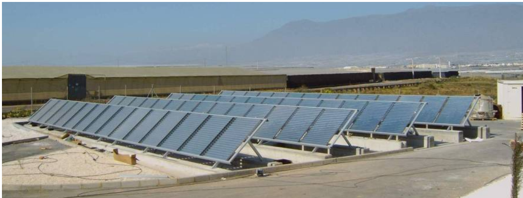
Figure 3.6. Solar collector field of the Albaida plant in Almeria.
