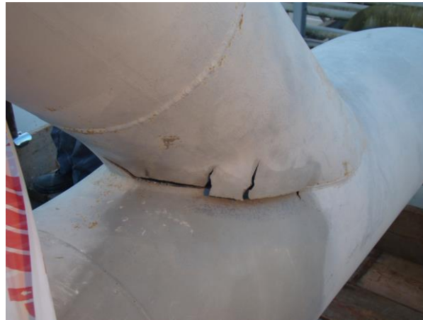
Figure 4-13. A failure occurred during blowdown (taken from Swindell, 2013).
