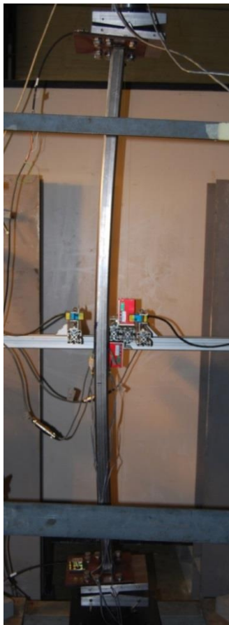
Fig. 4.34. Overall flexural buckling failure of specimen S3 – EC1.
