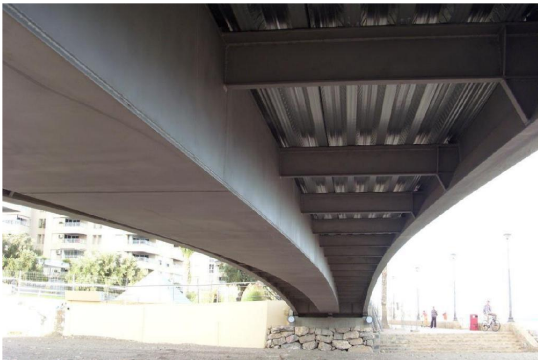
b) Bottom structural view of the pedestrian bridge. (Image by VALTER, Valenciana de Estructuras)
