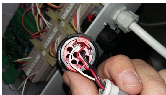
Figure A1.1: Image of the 4 wires Pt100 connected to the harness. Image source: A. Gilabert
