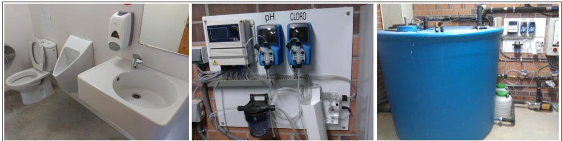
Figure 6.4 Automatic tap and waterless urinal in the bathroom (left), chlorination system (centre) and secondary tank with chlorination system (right).
