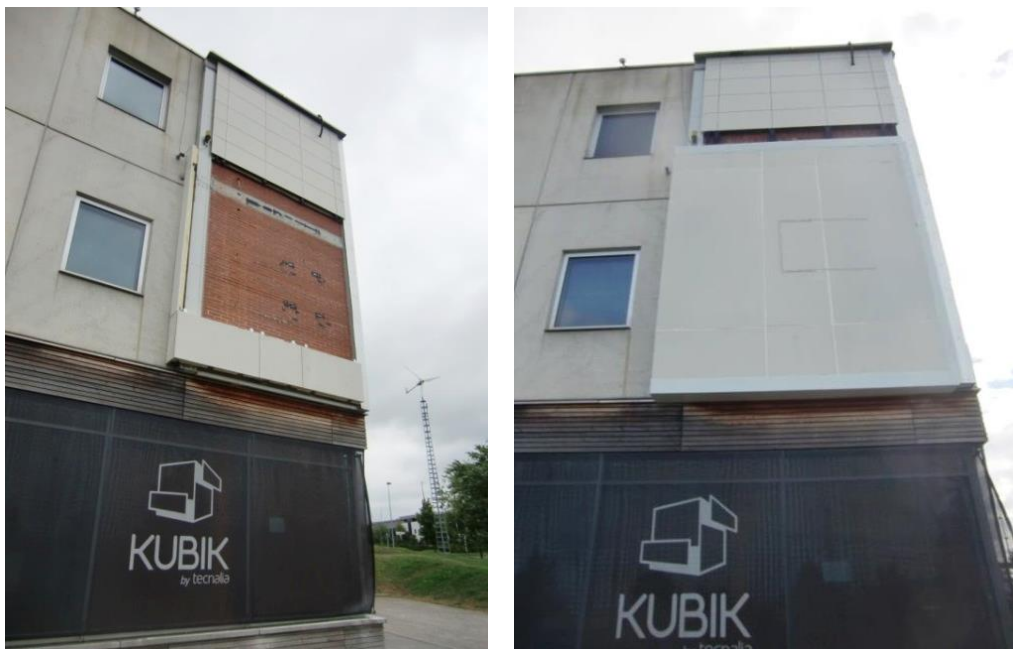
Figure 1: Test area at first floor of west-facing façade in KUBIK facility: (a) original brick wall before installation; (b) ETIXc prototype installed.
