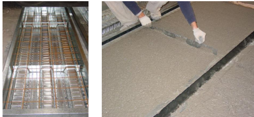
Figure 3.3 Crack inducer inclusion as part of the preparation of the laboratory specimen
