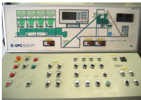
Mix machine Controller
