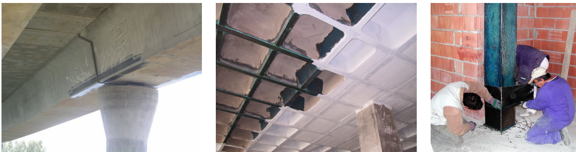
Figure 1.2. Application of composite materials for retrofitting concrete structures such a bridge deck, a slab or a column. (Bettor MBT, Degussa Construction Chemicals España, S.A.)
