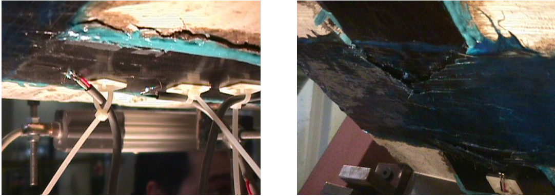
Figure C.62. Peeling of the laminate between two cracks in the concrete interface. Rupture of the external anchorage at the plate end.
