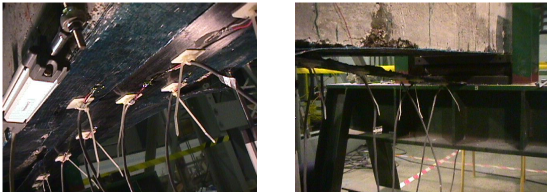
Figure C.79. Pultruded laminate bonded on the top of a wet lay-up lamina. Laminate peeling of both pultruded and wet lay-up laminates.
