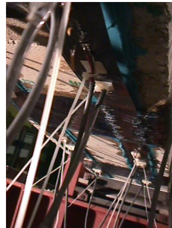
Figure C.54. External anchorages applied on Beam 2/B. Laminate debonding followed by the slip of the laminate up to the rupture of the external anchorage nearest to midspan.
