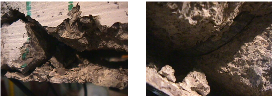
Figure C.73. Both laminates peeled-off with the detachment of the concrete cover, leaving some visible stirrups.
