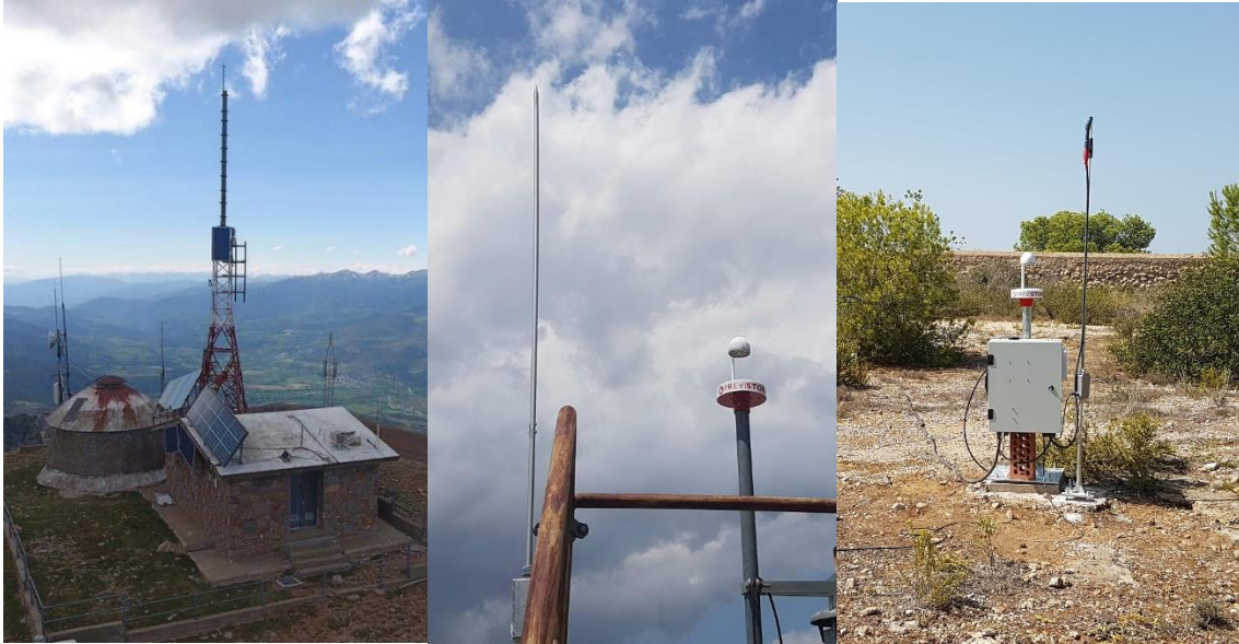
Figure 3.8 - Sharp grounded rod installed in the two setups: rooftop (left) and flat-ground (right).
