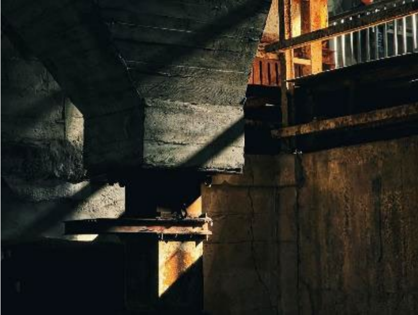
Figure 4.7 Internal structure of Huaxin Cement Plant
