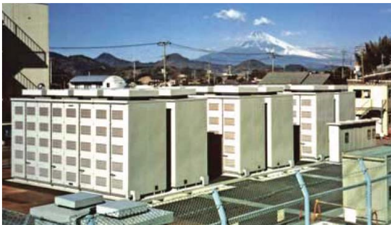
Figure 3.17 NaS batteries installation at TEPCO site. Source: POWER Magazine.
