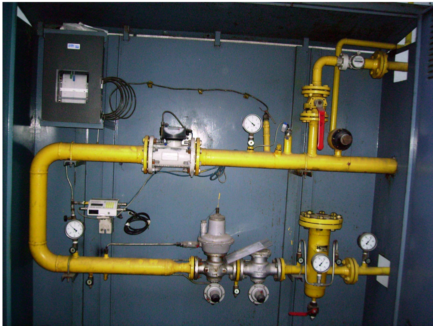
Figure 5.12 Mill B gas meter (elster ETM) and its converter (EK 88)
