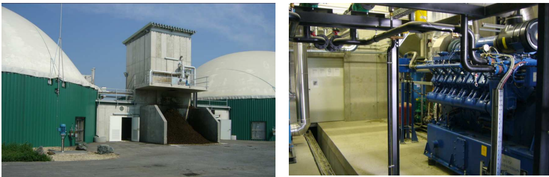
Figure 8.9 Biogas plant in Ethern Austria. On the left side, a view of the two digester tanks. On the right side, a biogas engine of 1 MWe.
