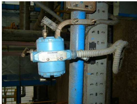
Figure 5.11 Steam flow meter Mill A. Vortex type
