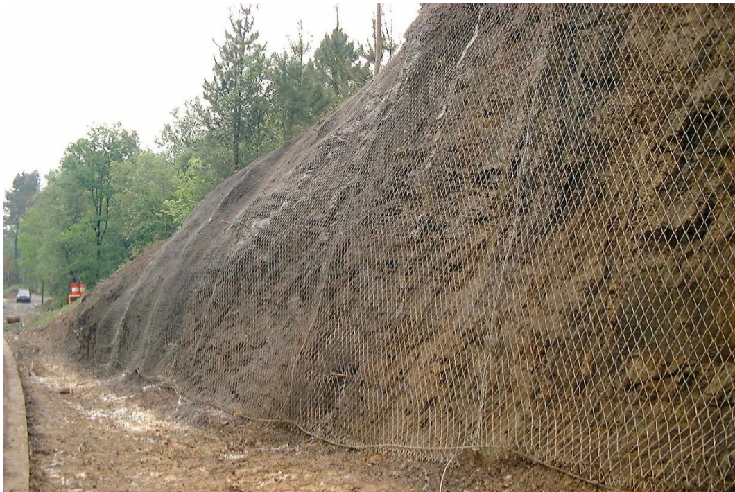
Figure 3.- High-resistance flexible system. Wire mesh anchored in a soil slope.
