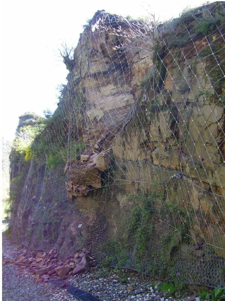
Figure 1.- High-resistance flexible system. Cable net anchored in a rock slope
