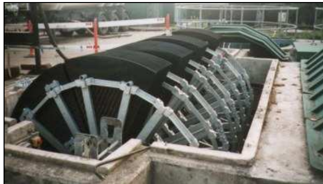
Figure 1.3 View of a rotating biological contactor
