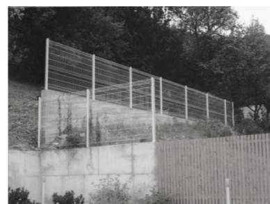
Figure III.20: the case of clear demarcation of boundaries with no overlap area. Outskirts of Bratislava, Slovak Republic.
